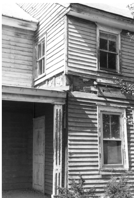
Detail showing framing and brick fill on south corner of Section A. 1984 photograph.
